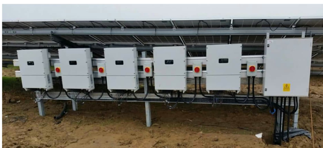
Plate 2-3: Typical String Inverter Installed Next to Solar PV Panels (prior to reinstatement)
