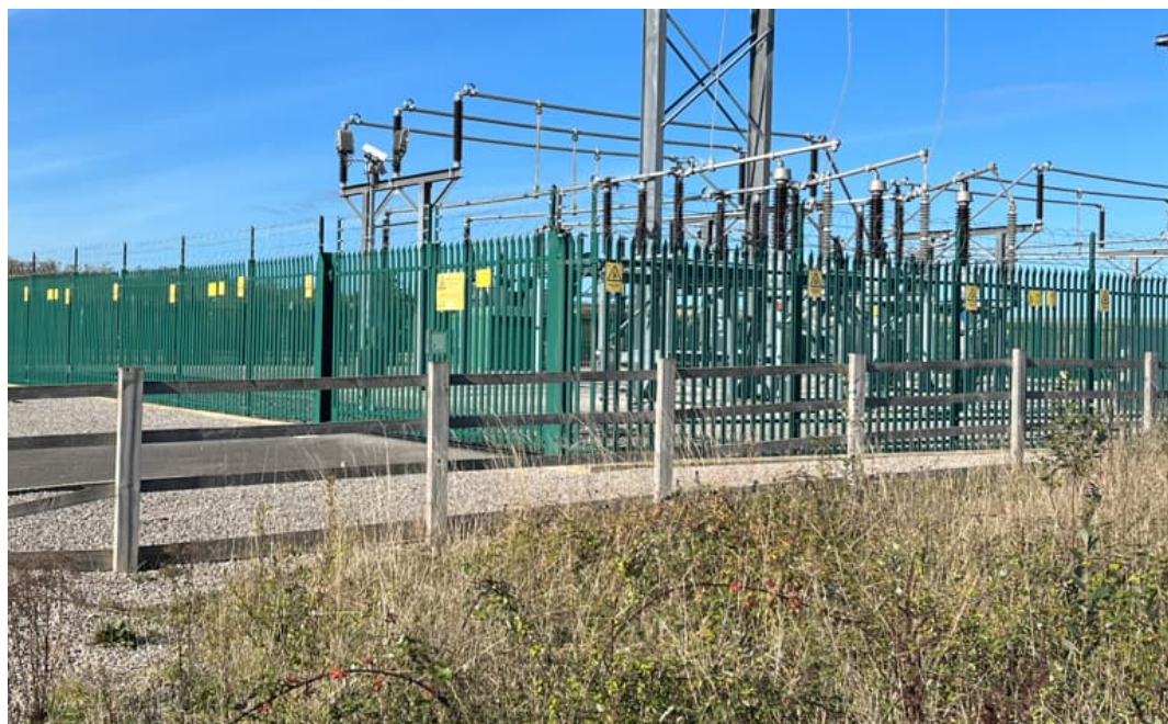
Plate 2-5: Example On-Site Substation showing Infrastructure and Fencing
