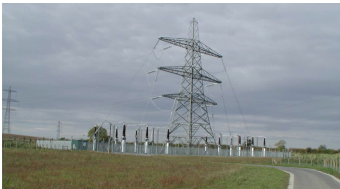
Plate 2-6: Example Line Drop On-Site Substation
